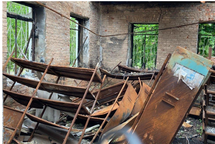
Barvinkove, Kharkiv region. Village library destroyed in March 2022
