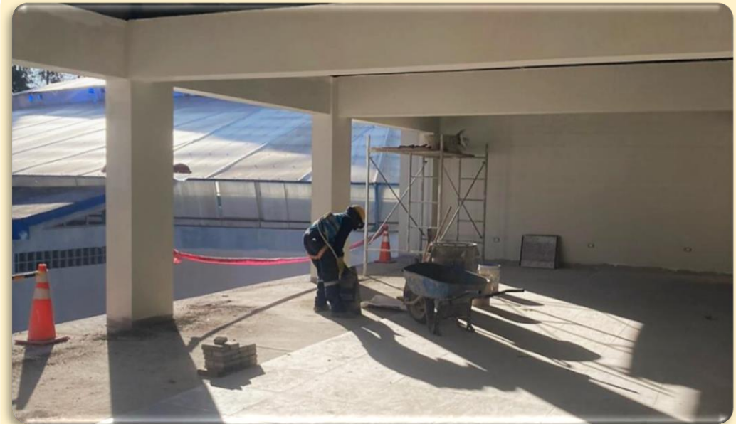
Progress of investment work – Municipal Library of the district of Poroy, province and department of Cusco.
